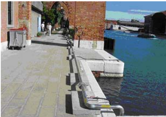
Figure 5 . The main distribution conduit
